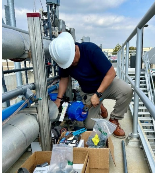
Sample pump installation for routine monitoring of biological tanks at the NIC demonstration facility
