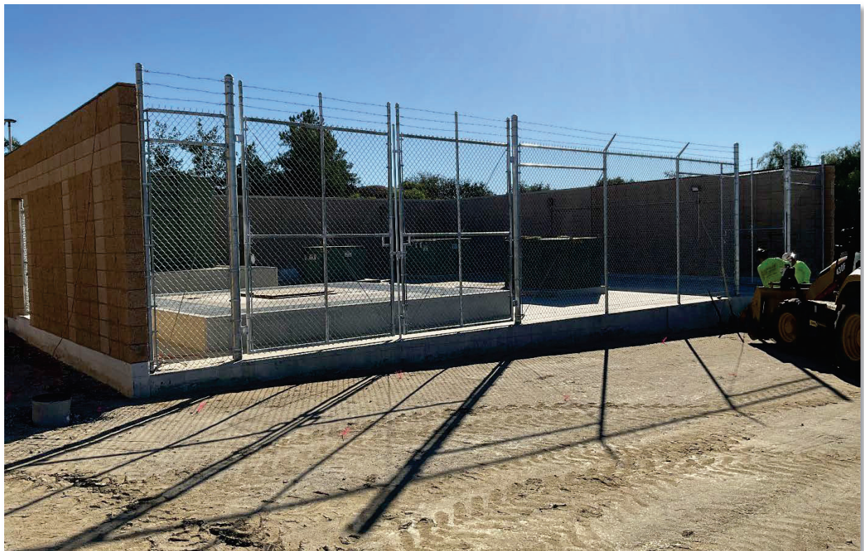
Expanded Riverside Public Utility switchyard for the second utility service for the Mills plant
