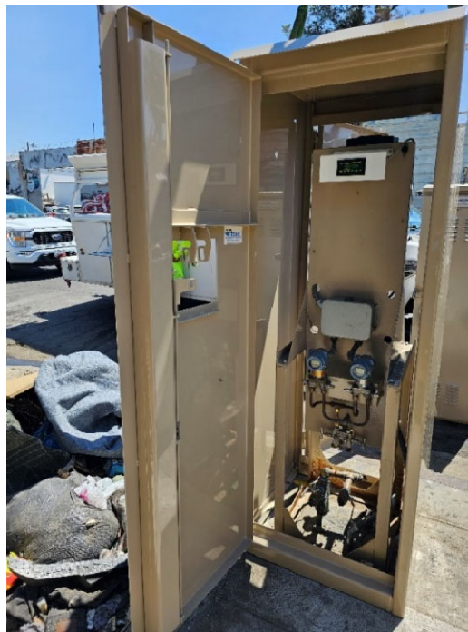
Automated Meter Reading (AMR) billing meter cabinet
