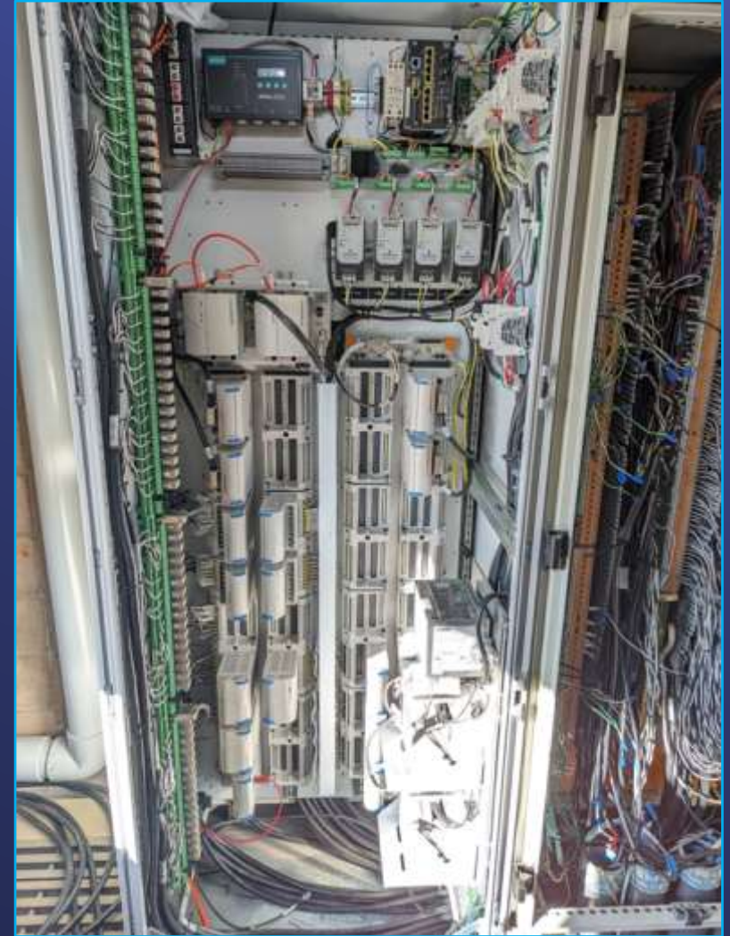
Mills Control System Upgrades
