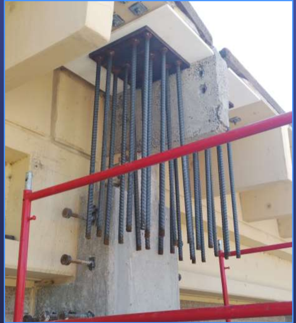
Installation of Rebars and Post-Tensioning Bars for Seismic Reinforcement of the Columns
