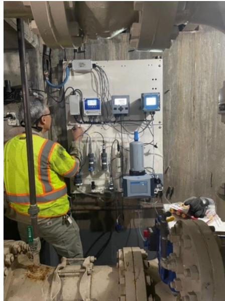
Staff working on a water quality panel at the Beverly Hills Pressure Control Structure
