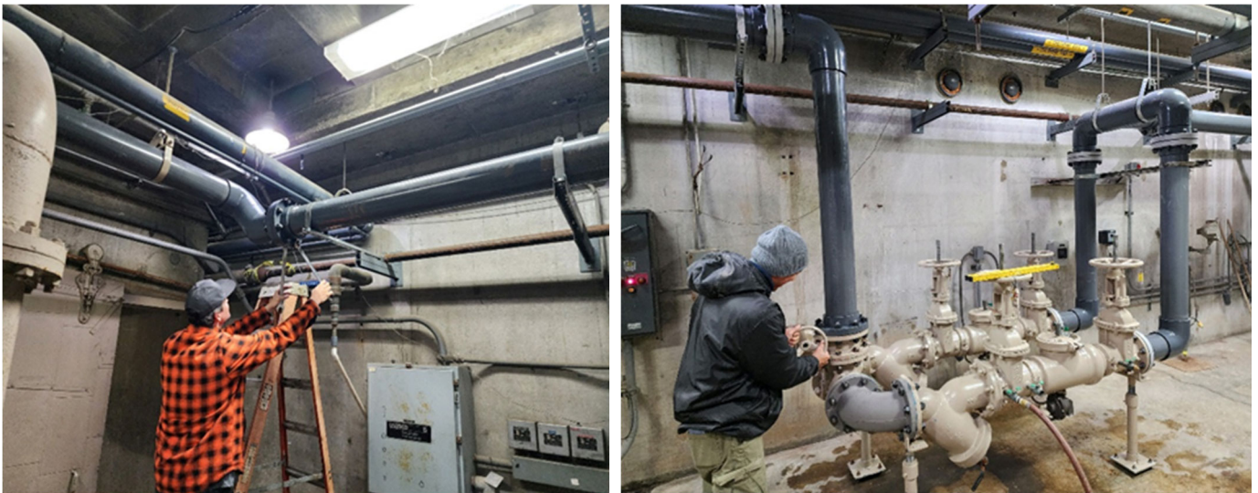
Staff assembling supply piping (left) and checking for leaks (right) at the Weymouth plant
