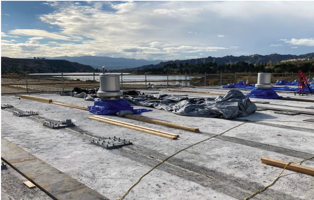
Installation of steel reinforcement plates on roof of the Foothill Hydroelectric Power Plant building
