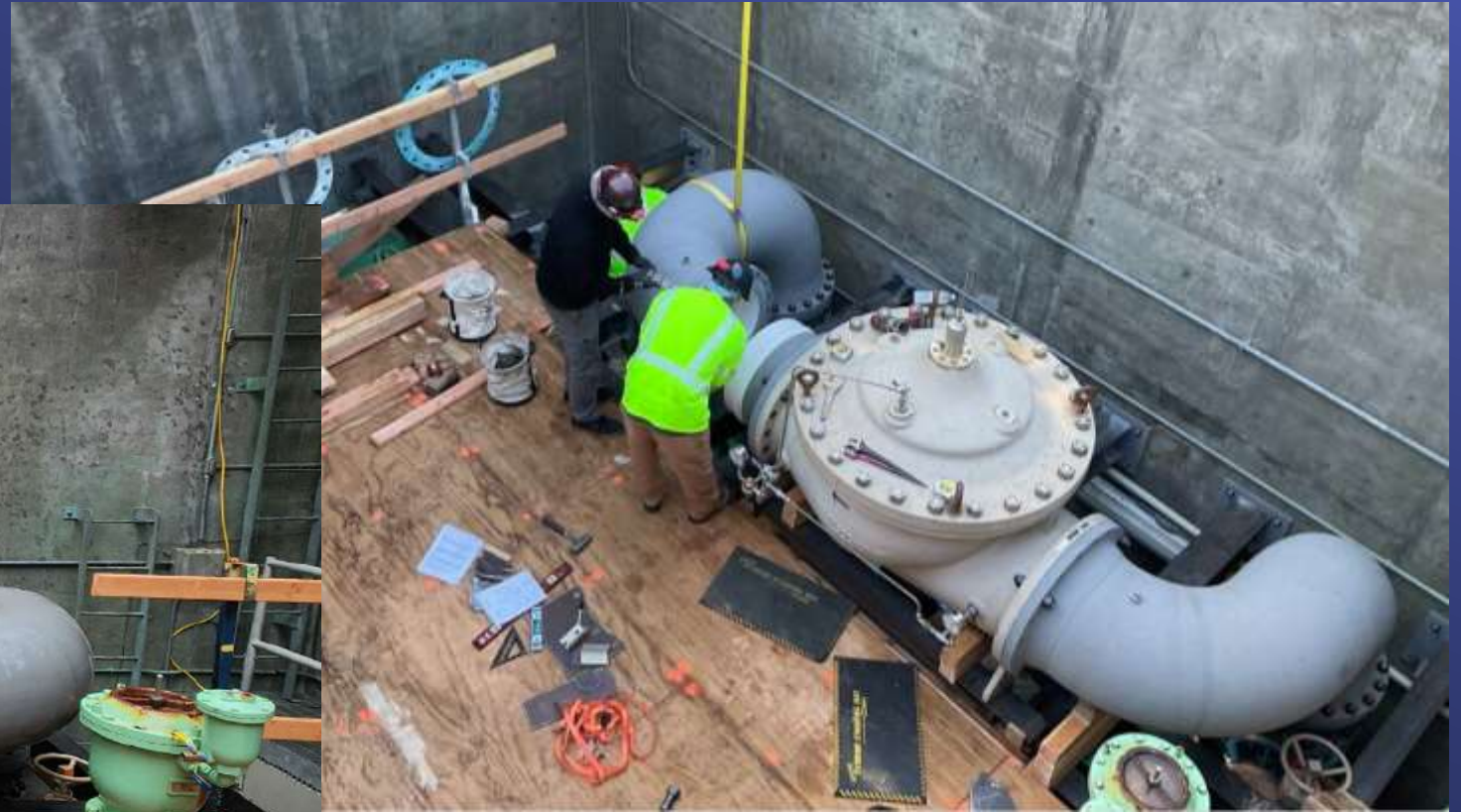
24-inch Cla Valve installed in 66-inch valve vault near OC-88
