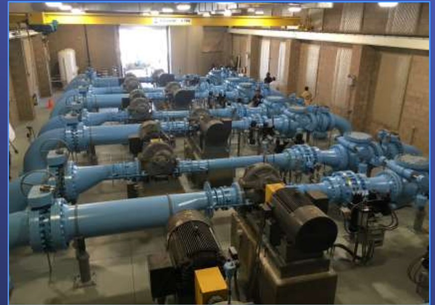
SBVMWD's Foothill Pump Station
