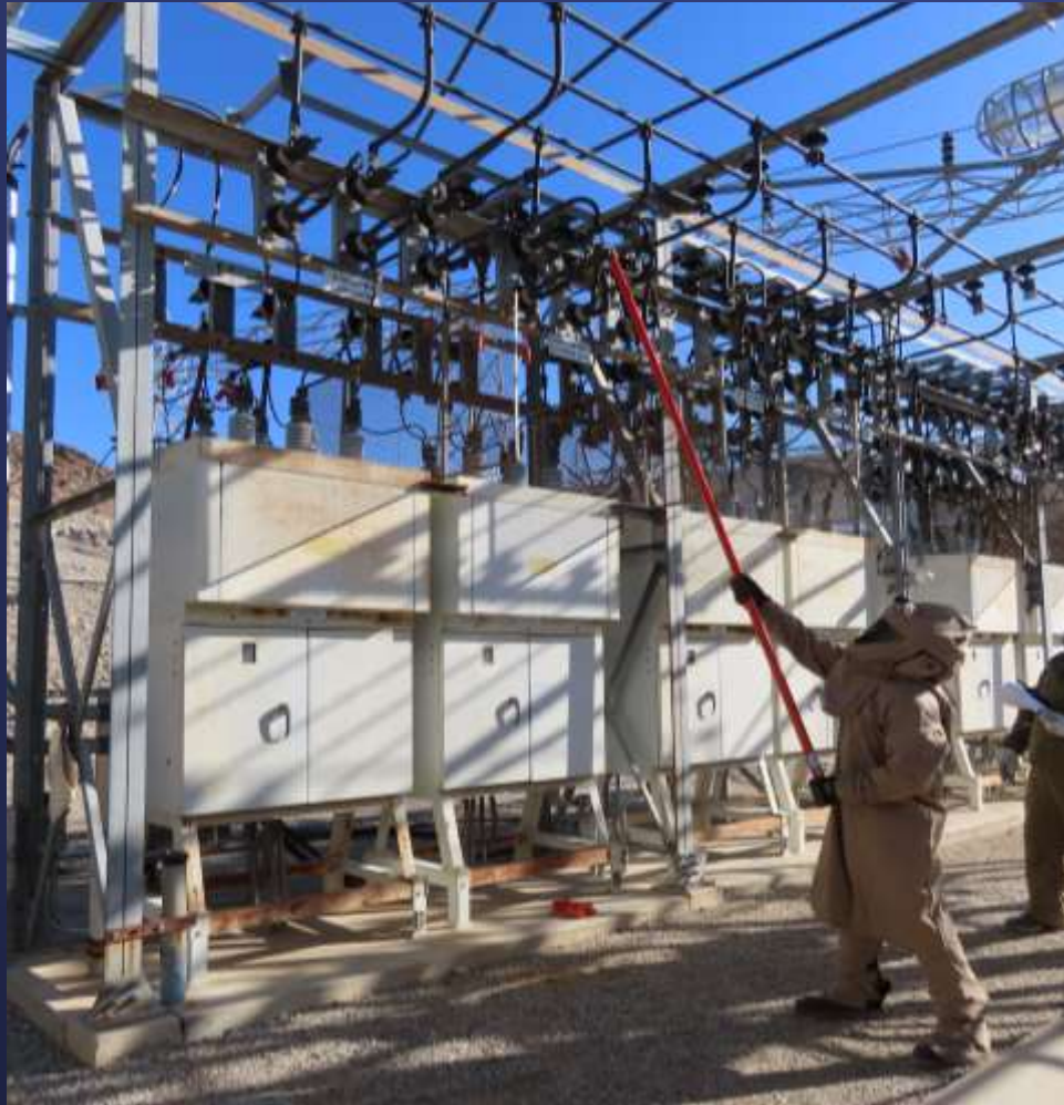
Existing 2.3 kV SL&P Switchrack
