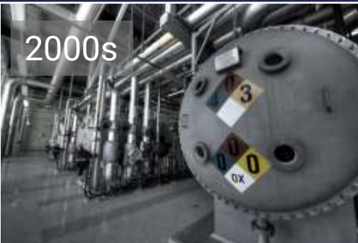
Ozone retrofit of treatment plants
