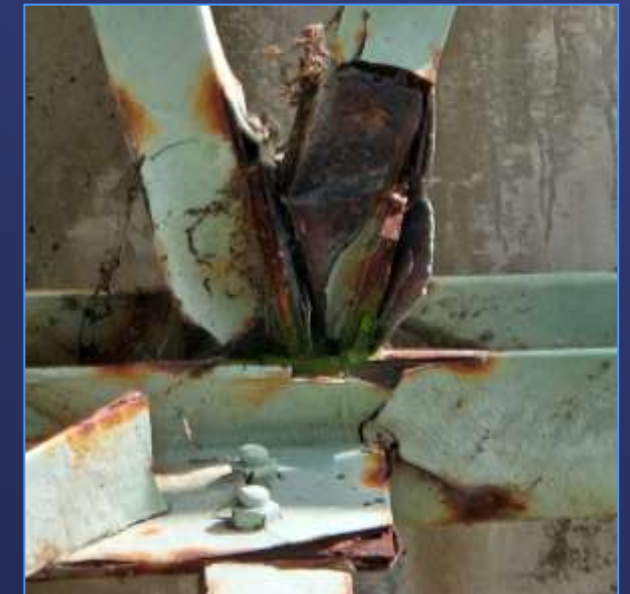
Corroded Structural Members
