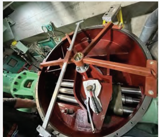
Discharge valve actuator open during functional testing
