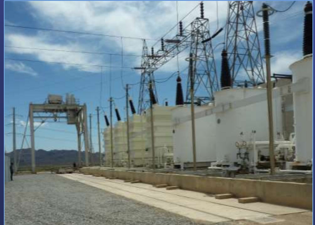
Hinds Pumping Plant
