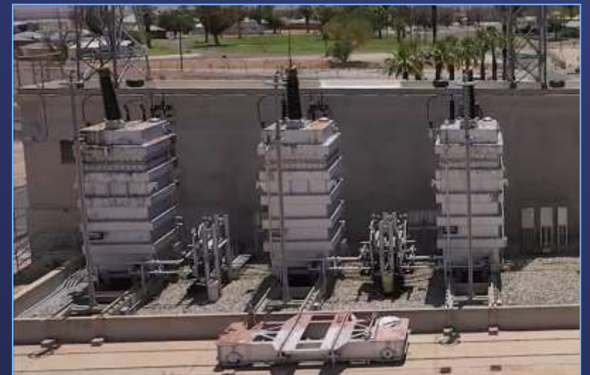
Iron Mtn. Pumping Plant
