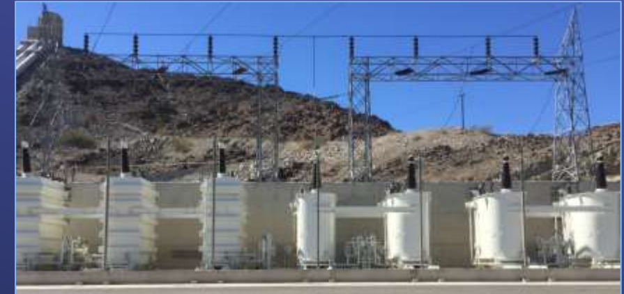
Eagle Mtn. Pumping Plant
