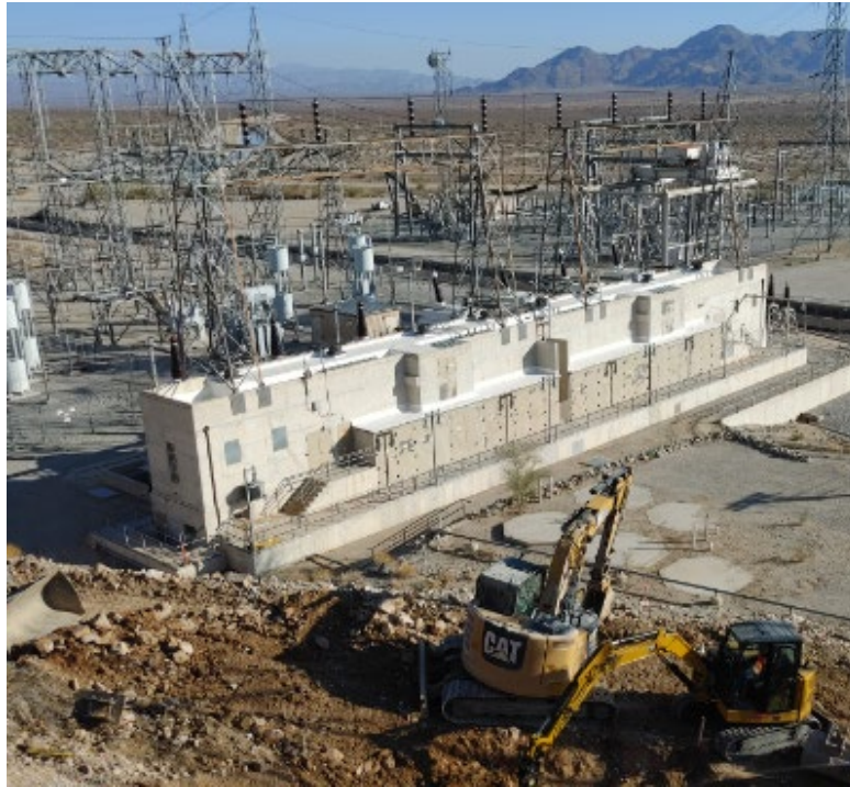
CRA Domestic Water Treatment System — Installing underground ductbank and precast accessways at Hinds
