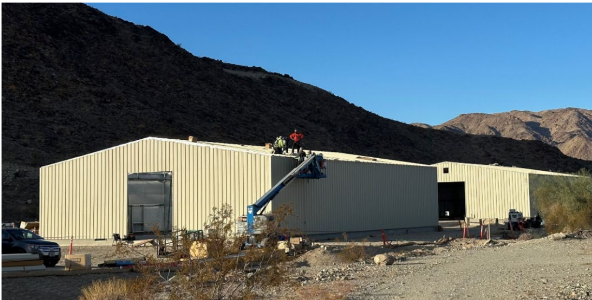
Eagle Mtn. Storage Building — Contractor Installation of Roof Paneling on New Building
