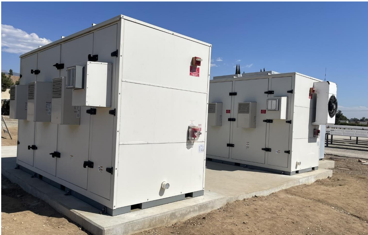
BESS enclosures at the Weymouth plant
