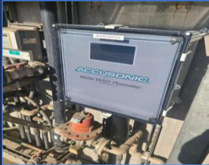
Weymouth Rapid Mix Influent Flow Meters Upgrade
