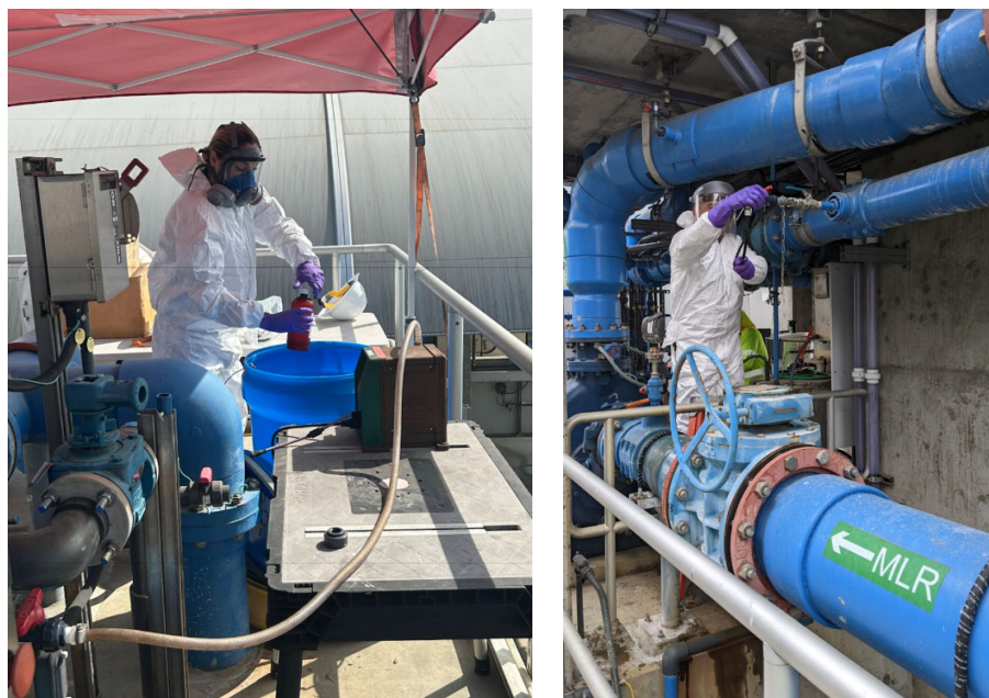
Staff preparing solution for VOC spiking test (left) and performing preventative maintenance on the membrane bioreactor system (right) at the Napolitano Center
