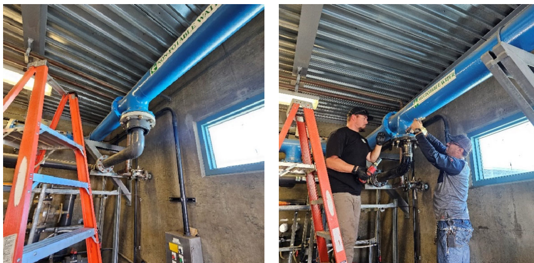
PVC pipe section before replacement (right) and staff installing carbon steel pipe at the Skinner plant
