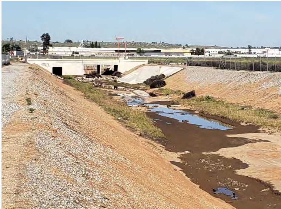
Photograph 8. Lateral B where it transitions from concrete- to dirt-channel, with evidence of existing erosion, regular vegetation clearing, and debris. Located approximately 6,000 feet downstream of Discharge Point B.
