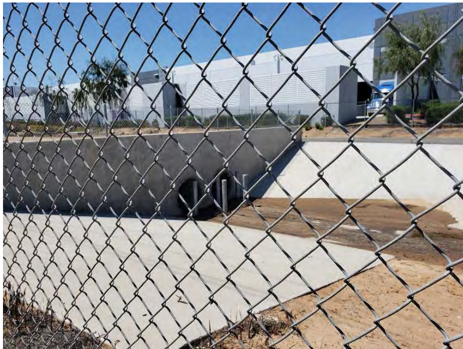
Photograph 6. Discharge Point A (concrete-lined channel) located west of I-215 and north of Harley Knox Boulevard.
