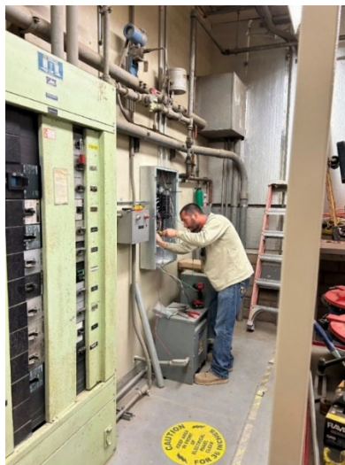
Staff replacing electrical distribution panel in the Mechanical, Electrical, and Fleet shop at the Skinner plant
