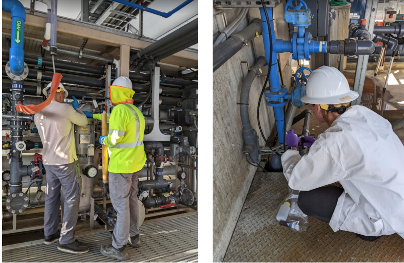
Staff replacing cartridge filters ahead of reverse osmosis system (left) and collecting samples during VOC spike testing (right)
