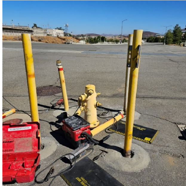
Replacement of bollards protecting fire hydrant with new, taller bollards for increased protection and visibility
