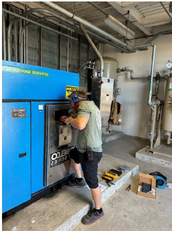
Staff installing Human Machine Interface (HMI) for interactive control and data related to the ozone contactor air compressor system
