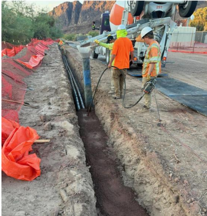
Gene Communications Upgrades— Placement of approximately 50 cu yd concrete for an electrical ductbank
