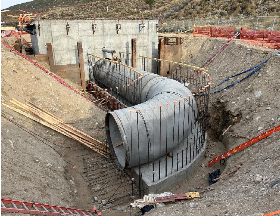
Inland Feeder Rialto-Pipeline Intertie—East 96 Inch Pipe to Inland Feeder—Looking West
