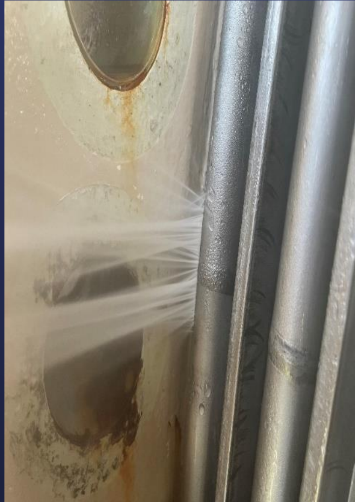
Initial leak on bellows joint
