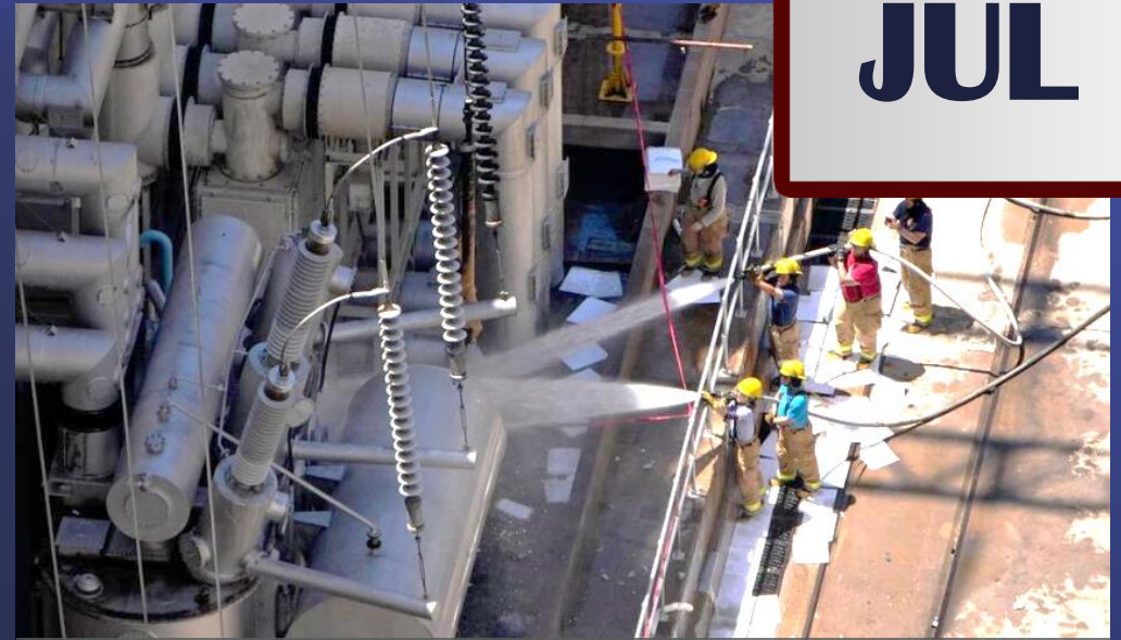
USBR fire crews quickly extinguish fire
