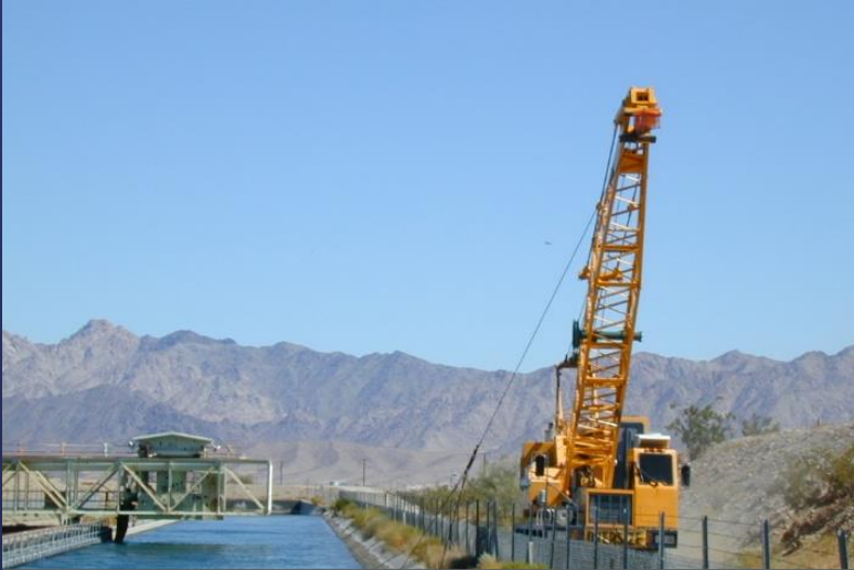
Cleaning CRA while operating
