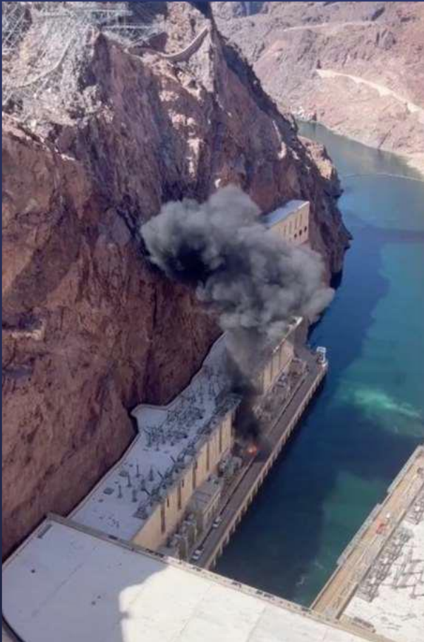
Explosion at Hoover Dam July 19, 2022
