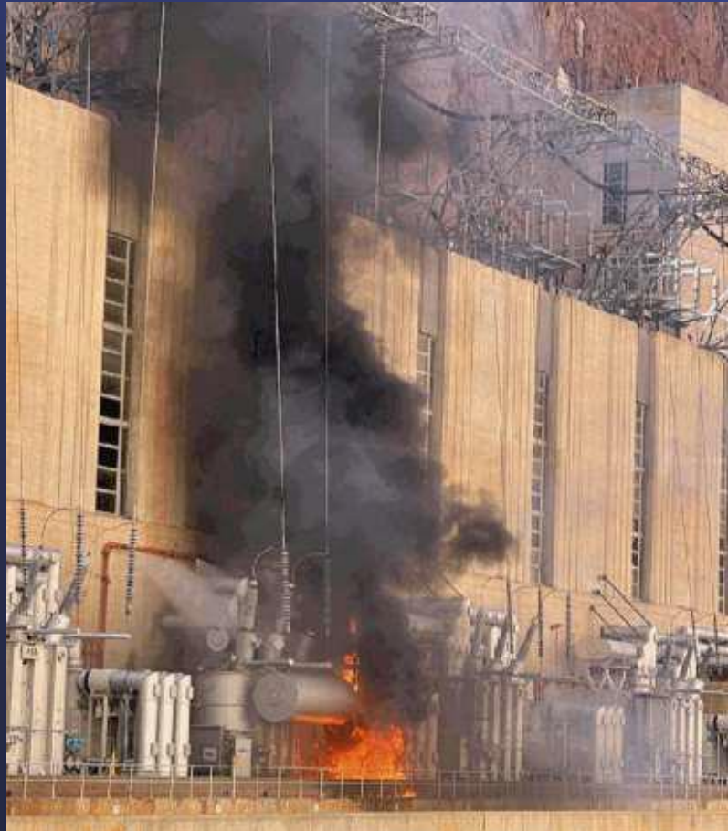
Transformer fire due to 230kV bushing failure
