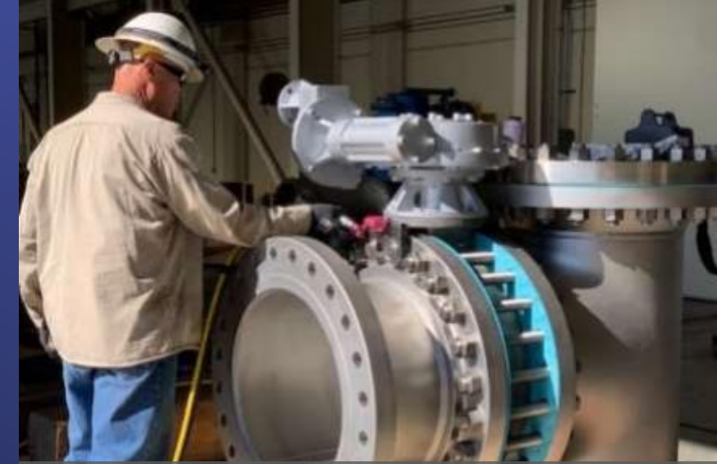
Branch tee for recirculation
