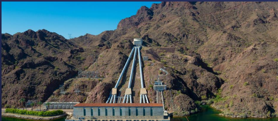
Intake Pumping Plant
