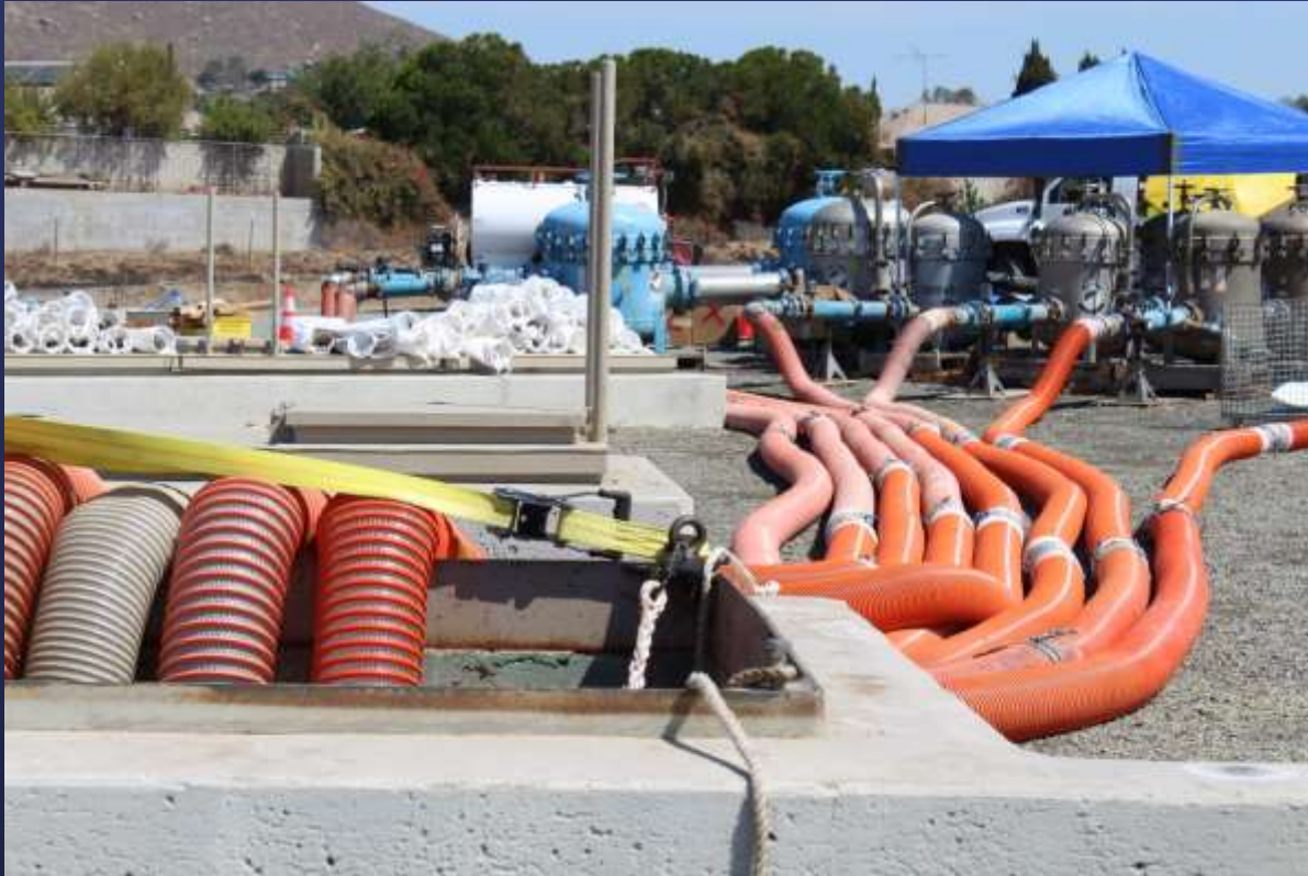
Quagga Mussel Filtration during Dewatering
