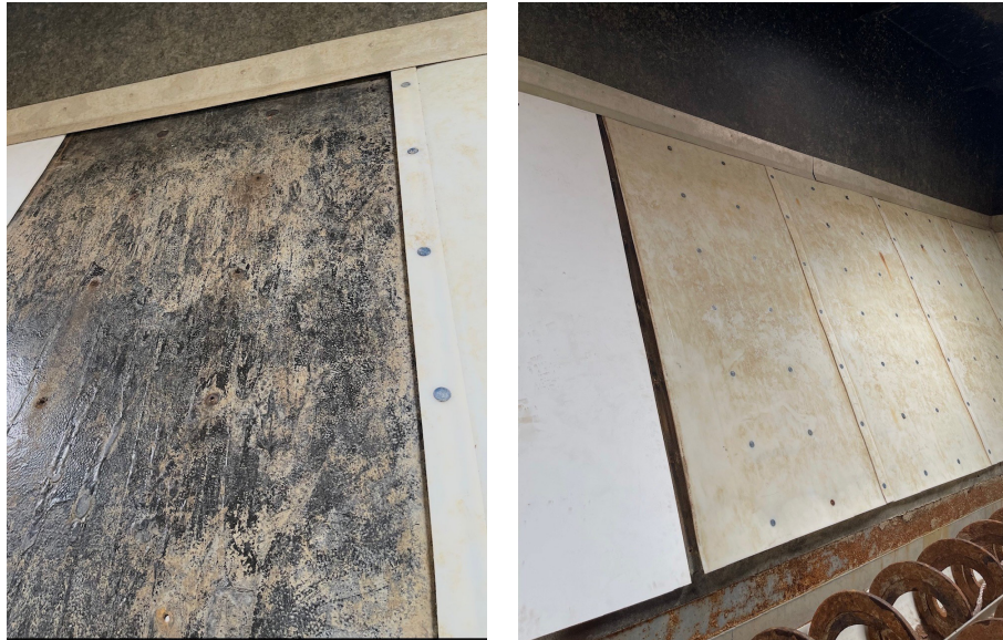
Failed Teflon panel (left) and the newly installed panel (right)
