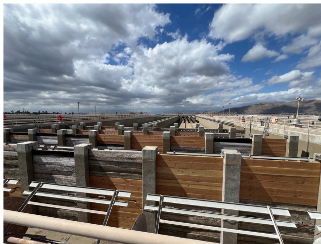
New flocculation basin baffle boards at Mills plant.
