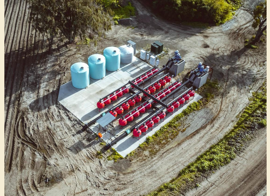
A drip filtration and pumping station — solar-powered
