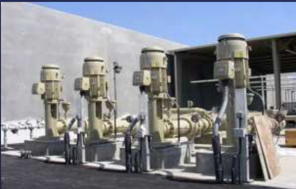
Irvine Desalter Project (IRWD)
