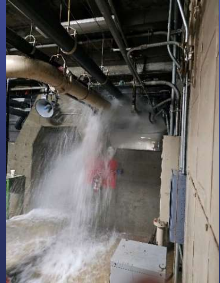
Weymouth Domestic Water Line Leak June 2024
