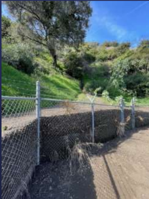
Sepulveda Feeder Erosion – February Storms 2024
