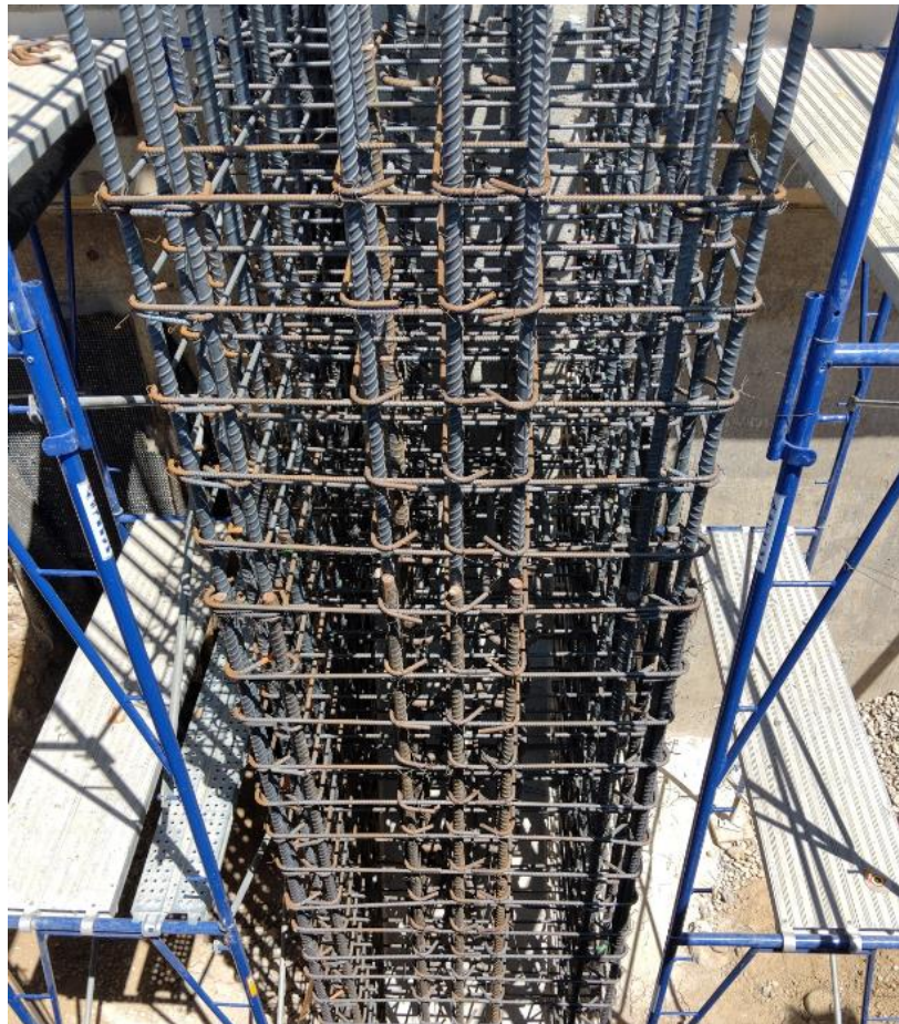
Foothill Hydroelectric Plant and Control Building Seismic Upgrade— Rebar Placement at Hydroelectric Plant Column
