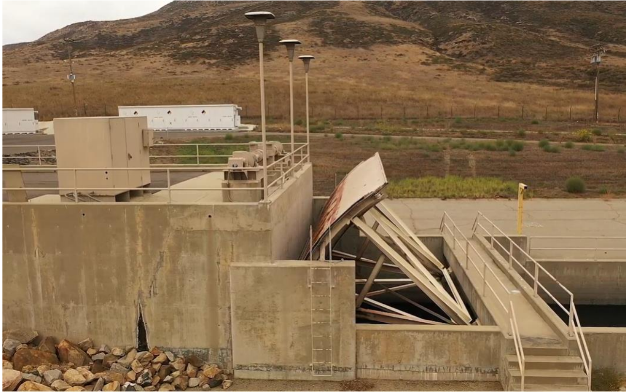
San Diego Inlet Canal to Lake Skinner Reservoir Radial Gate V-06
