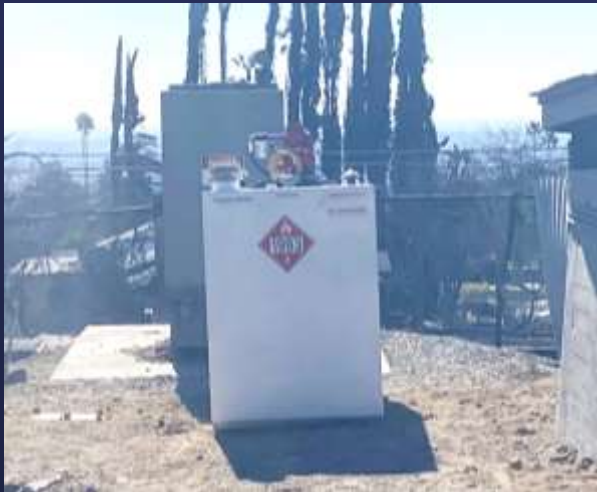
1,000-gal fuel tank for standby generator support
