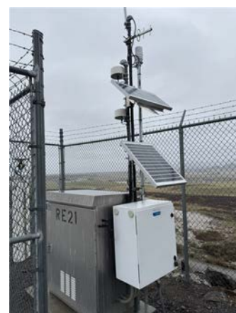
New monitoring equipment at Diamond Valley Lake
