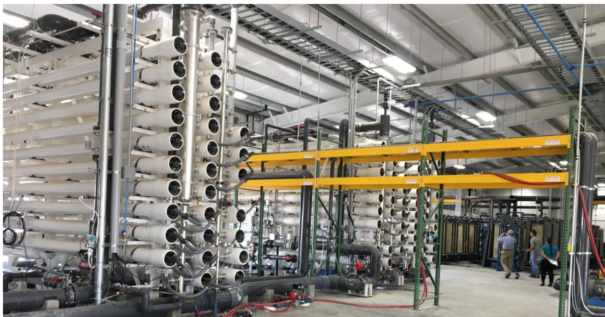
Figure 3.11 One-Million-Gallon-per-Day Mineral Recovery Facility in El Paso, TX (Enviro Water Minerals)
