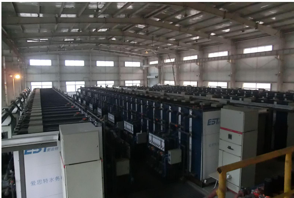
Figure 3.7 Power Generating Facility in China Reported to be Using CDI to Desalinate Reclaimed Water (Courtesy of estpure.com via web.archive.org)
