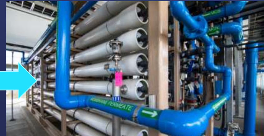
Advanced Water Treatment
