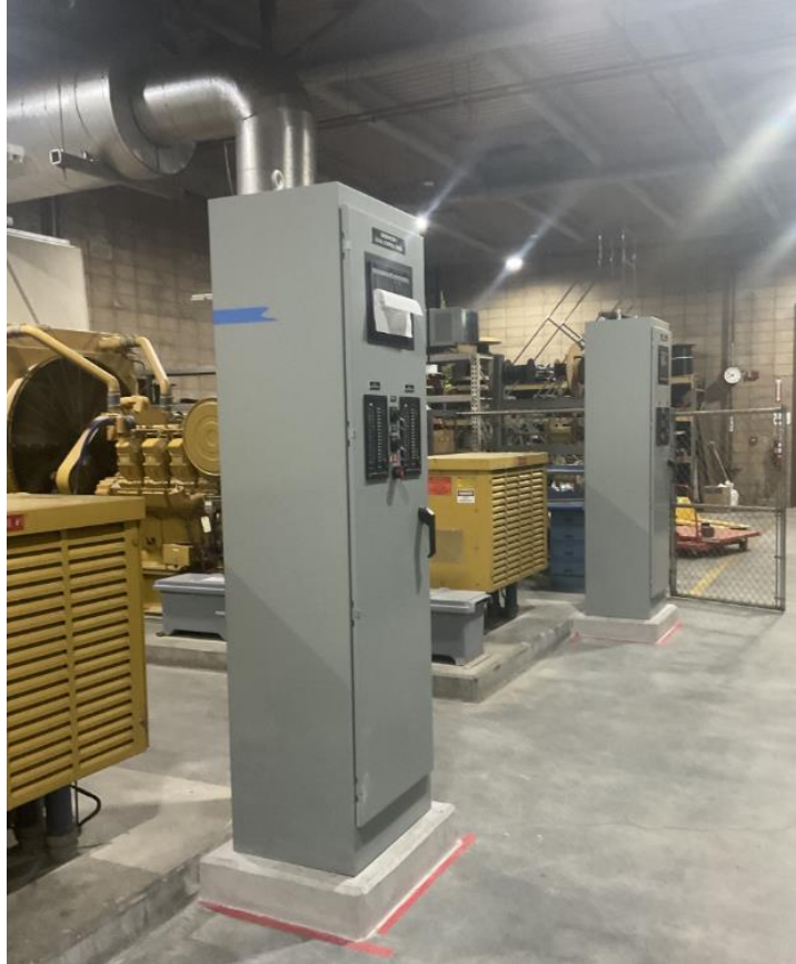
Mills Electrical Upgrades, Stage 2—New Control Panels Installed in the Engine Generator Building
