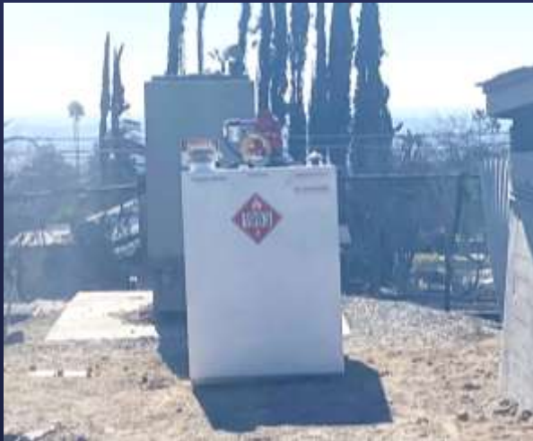
1,000-gal fuel tank for standby generator support
