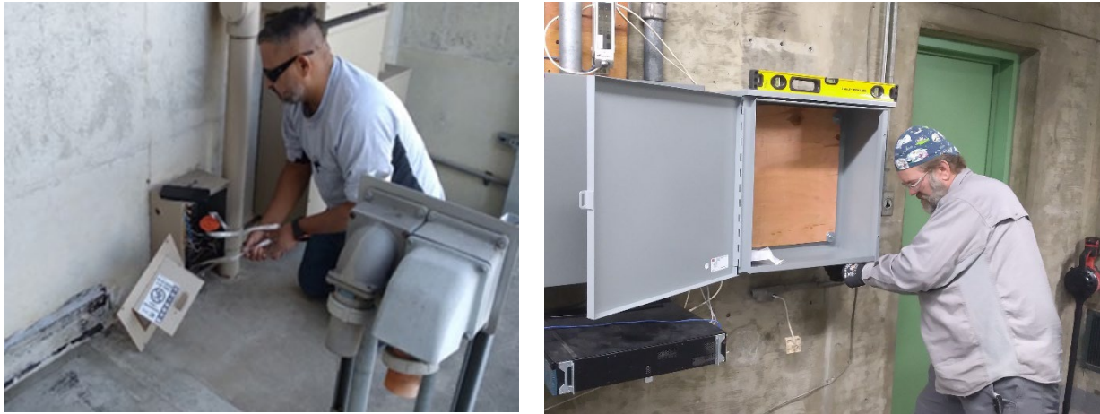
Staff installing pull rope (left) and mounting a new enclosure (right) at the Santiago Creek PCS
