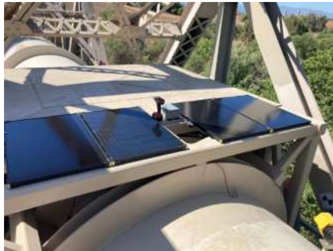
Solar panels for providing power to equipment monitoring sensors on the Upper Feeder's Santa Ana River bridge crossing
