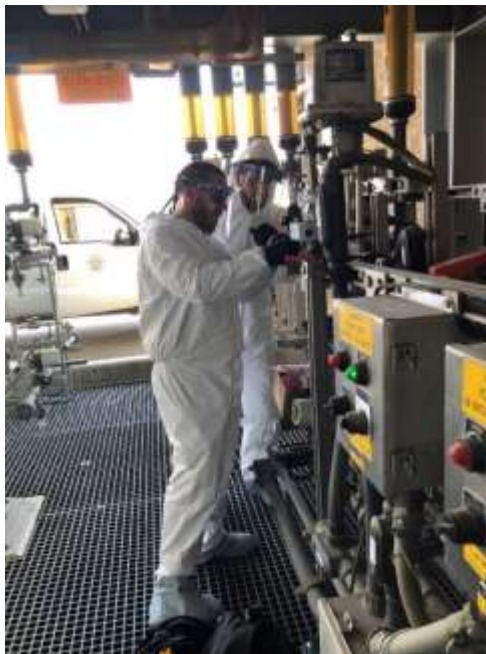
Staff installing a magnetic flow meter for measuring sodium hypochlorite at the Skinner plant
