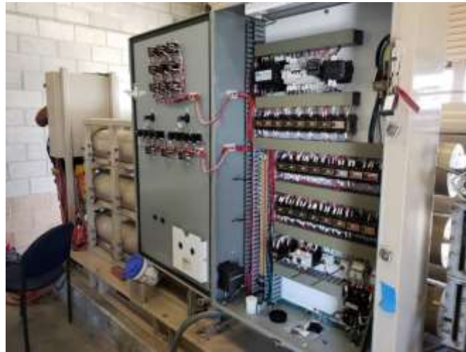
Finished control panel at the Lake Mathews junction shaft
