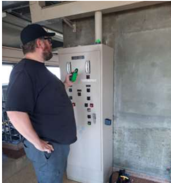
Staff verify wireless signal transmission of newly installed remote-control pendant for a backwash header valve at the Diemer plant
