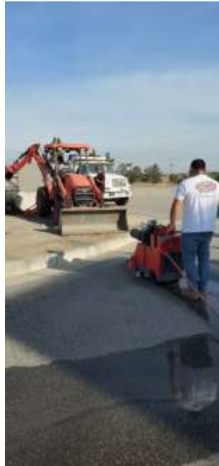
Staff saw cutting asphalt in preparation for pipe trench at the Skinner Plant
