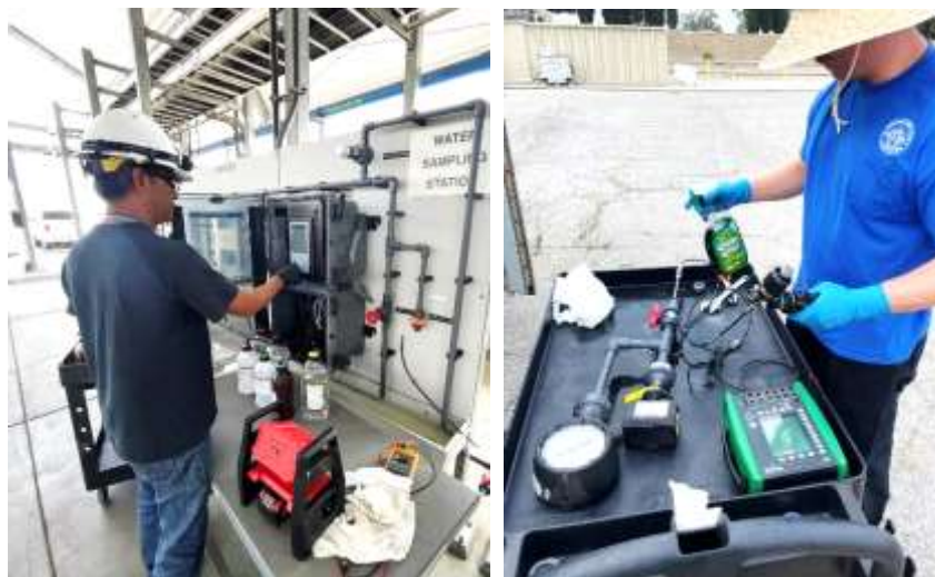
Staff troubleshooting instrument alarms (left) and calibrating pressures switches (right) at the Pure Water Southern California demonstration plant
