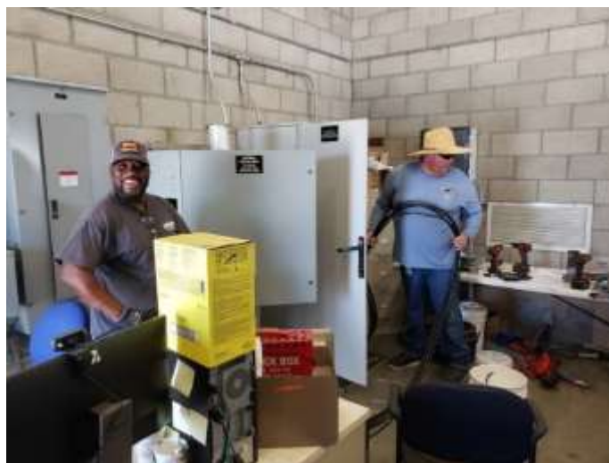
Staff pulling cabling for new gate controls at the Lake Mathews junction shaft
