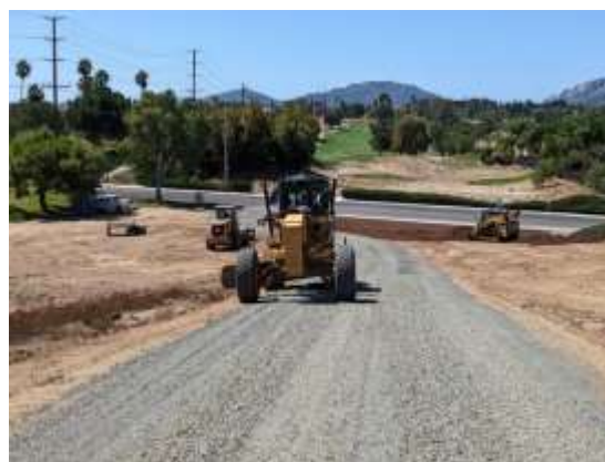
Staff completing road realignment for the San Diego 1 and 2 patrol road in Temecula
