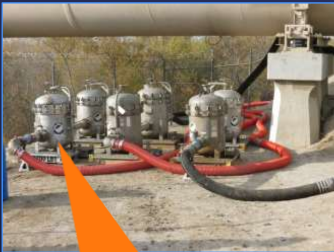
Quagga Filters for Dewatering
