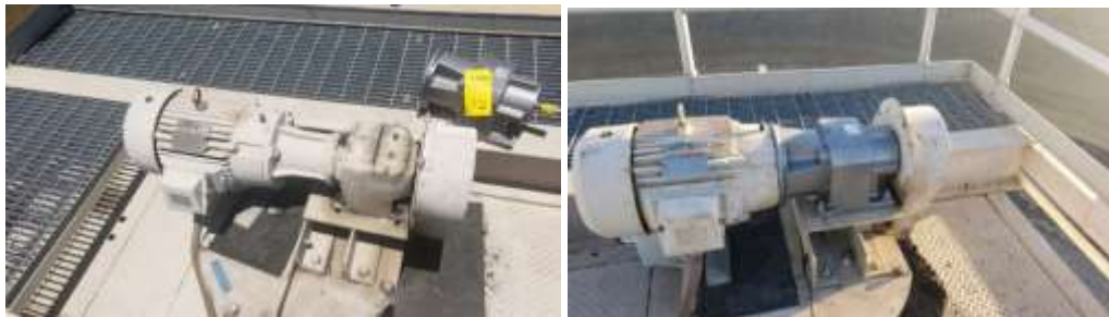
Failed (left) and new (right) gearbox at the Weymouth plant
