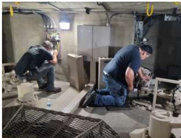
Staff adjusting the needle valve timing and control system at Etiwanda HEP
