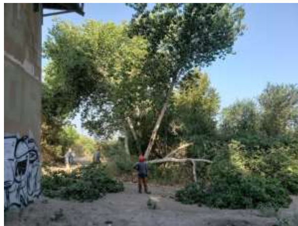
CalFire crews conducting vegetation maintenance in support of the Upper Feeder Santa Ana River Bridge Emergency Repairs Project
