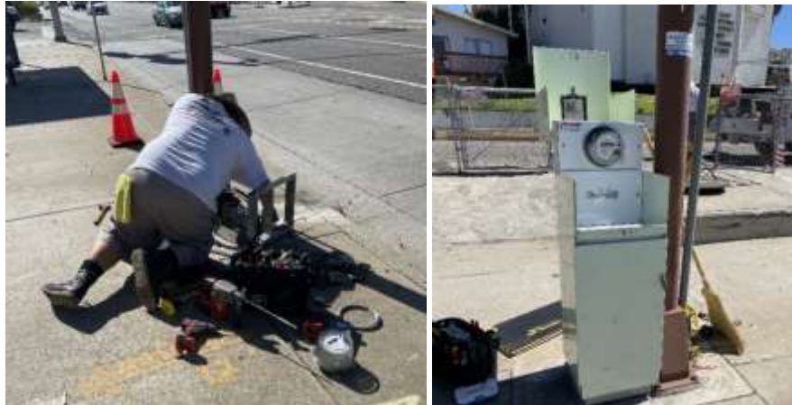
Staff preparing pedestal base (left) and new electrical service pedestal (right) at the Shenandoah PRS along the Culver City Feeder
