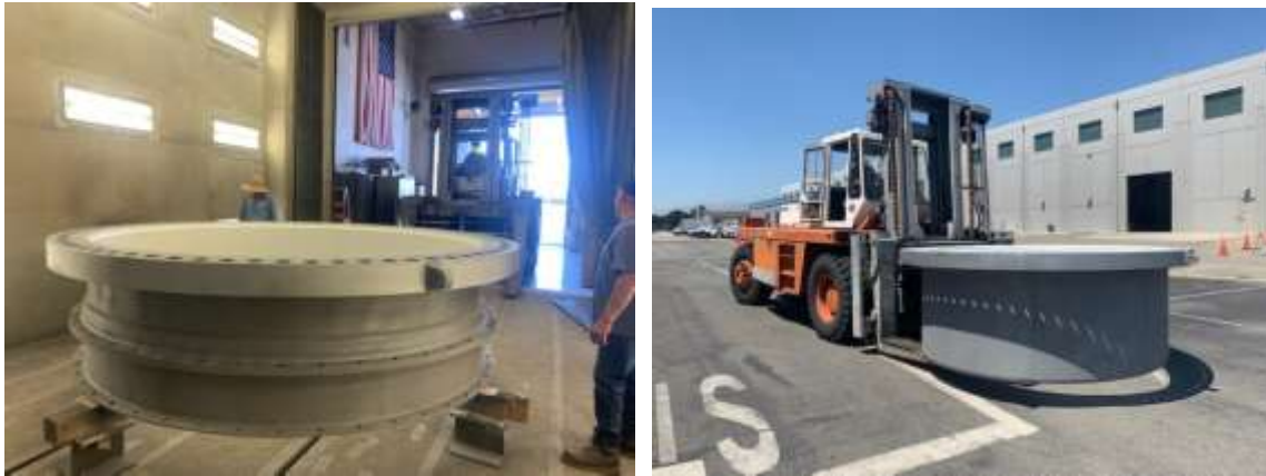
Coated upstream thimble (left) and downstream thimble (right) for the Upper Feeder repairs
