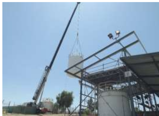
Staff using a crane to place the new sodium hypochlorite tank at Lake Mathews
