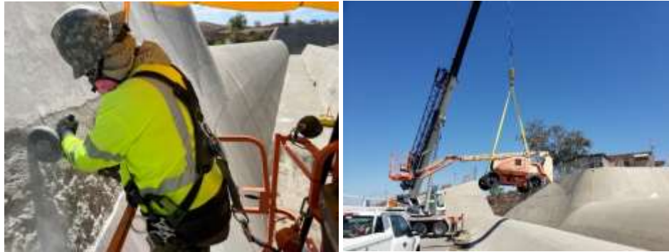
Staff removing loose and unstable material (left) and hoisting a man lift into the spillway channel (right) at Lake Skinner
