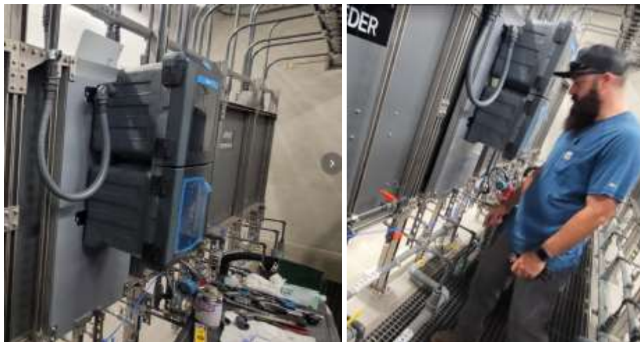
Staff installing sample line tie-ins to ammonia analyzers at the Weymouth plant
