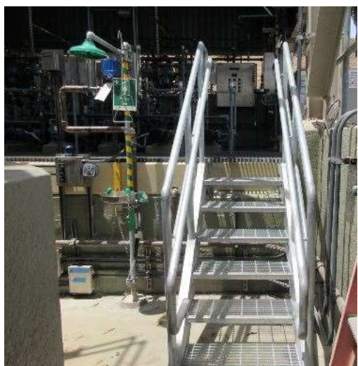
Garvey Reservoir Hypochlorite Feed System Replacement —New stairs for access to the containment area.
