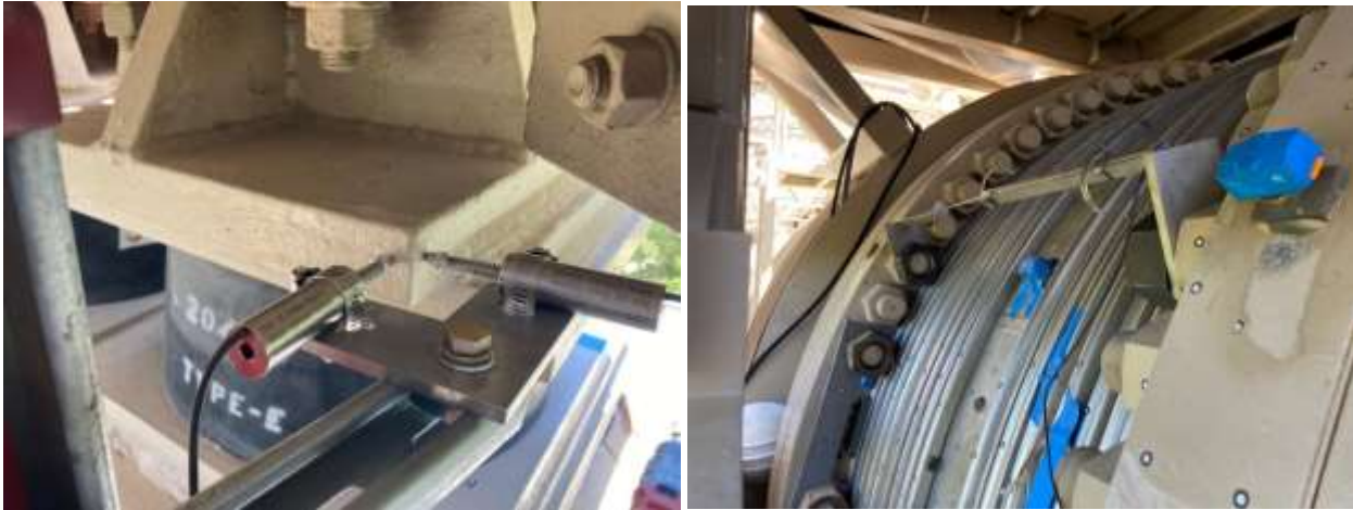
Equipment monitoring sensor installed at the Upper Feeder's Santa Ana River bridge crossing
