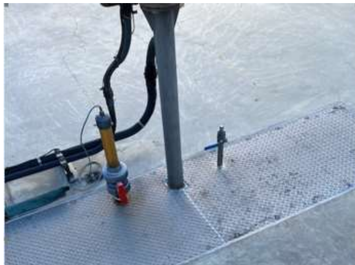
Ozone contactor afterbay gate hatch with a welded sample port at the Diemer plant
