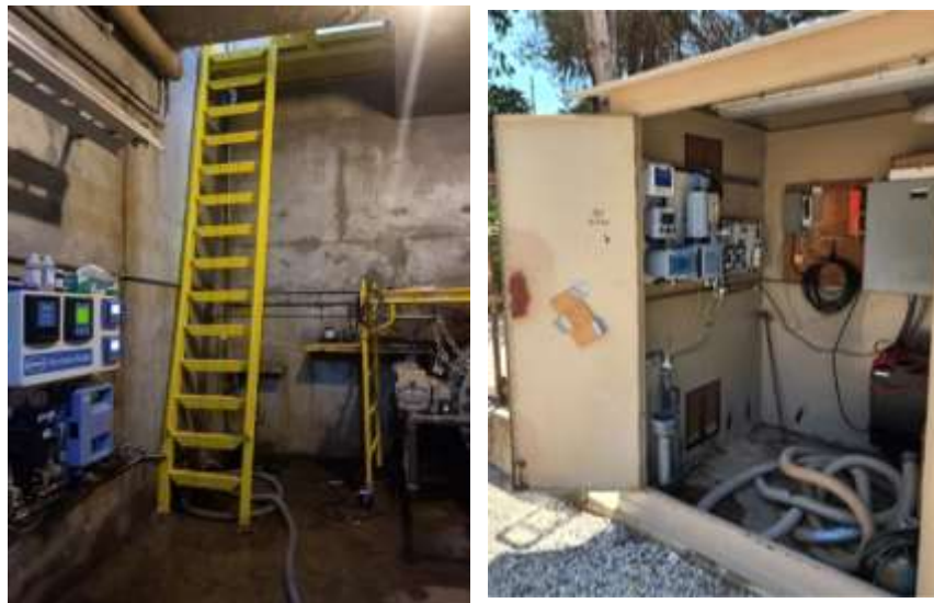
Obsolete underground water quality panel (left) and new ground-level water quality panel installed (right) at Palos Verdes Reservoir
